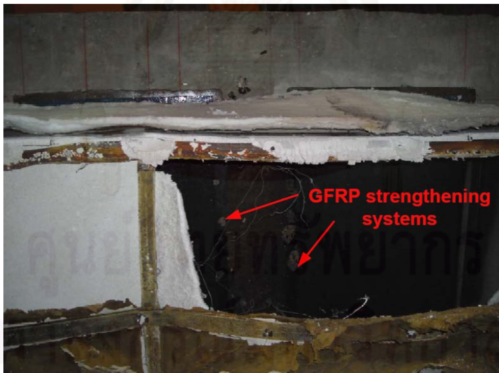
Figure 4.22 The GFRP strengthening system in specimen-1 after the fire test
