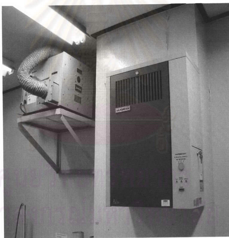
Figure 4.5 Humidifier in control room.
