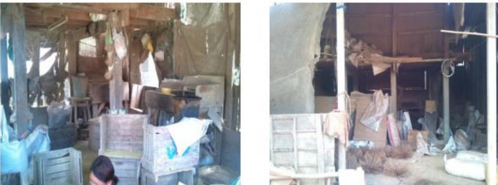
picture 30 - 31 Dust and incense powders spread on the floor and accumulated on the wall.
