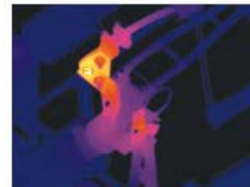
Infrared inspection helps to detect overheating parts, can avoid costly downtime and maintain plant efficiencies.
