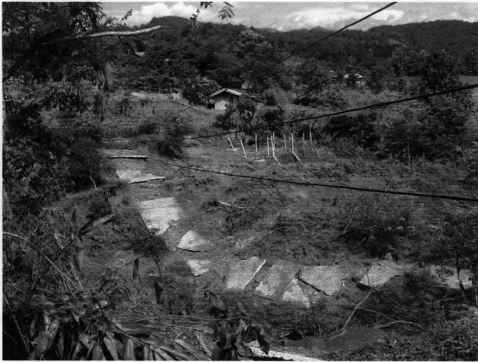
Figure 4.6 Landslide damaging the road, electricity poles, and house at Nam Phi Village, Thung Chang District, Nan Province.
