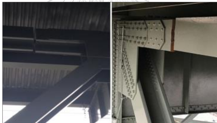
Fig. 1.2. A fracture occurred on a truss member of Turnpike Toll Bridge [6].
