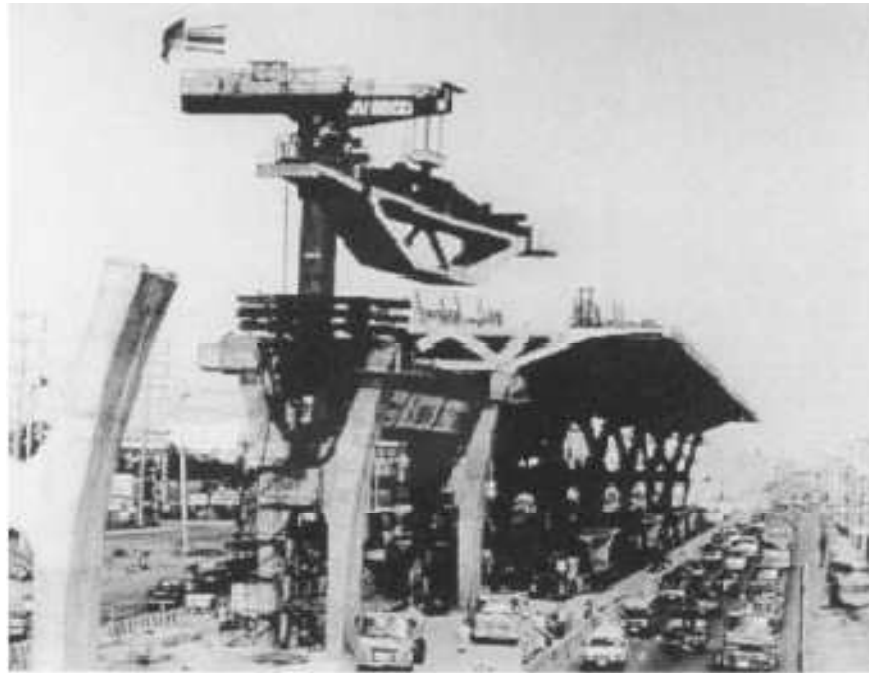
Figure 1.2: The BuraphaWithi Expressway Project in Thailand Using the Erection Gantry Method Source: Sauvageot, (2000)
