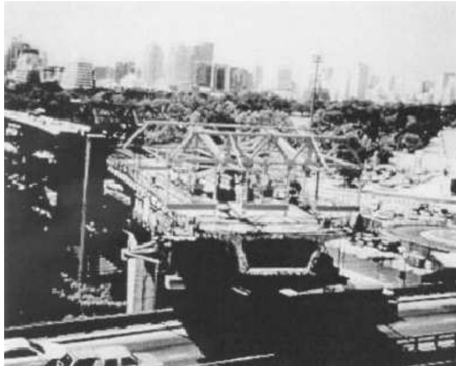
Figure 1.3: Construction of the Bangkok Mass Transit System Project with Long Span over Rama IV Flyover in Thailand Source: Sauvageot, (2000)
