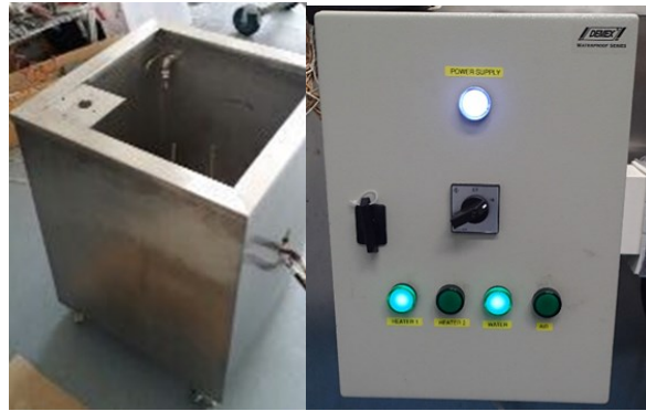
Figure 3. Photo of the water tank (left), control panel (right)
