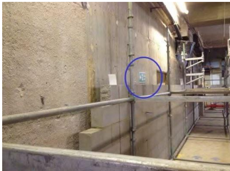
Figure 1.3 Obscure emergency exit sign on the construction site
