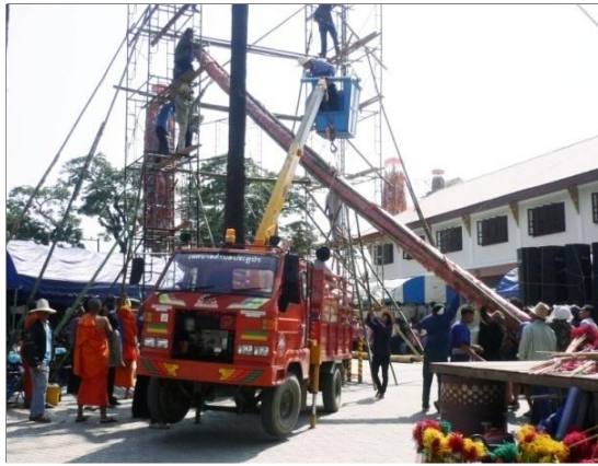
Figure 55 Crane trucks and scaffolds used in the assembly process instead of the traditional method Source: SP
