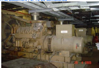
Existing Generator Rm. No : 1,2 "DALE" @ 625 KVA at Basement FL. To be demolished
