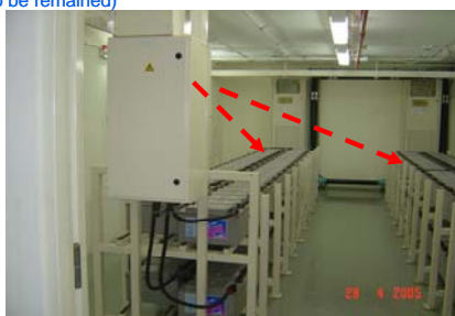
Existing Battery Rack No : 1 & 2 (To be remained)
