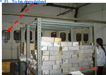
Existing HV-MDB2 Panel at substation Rm. 19 th FL. To be demolished
