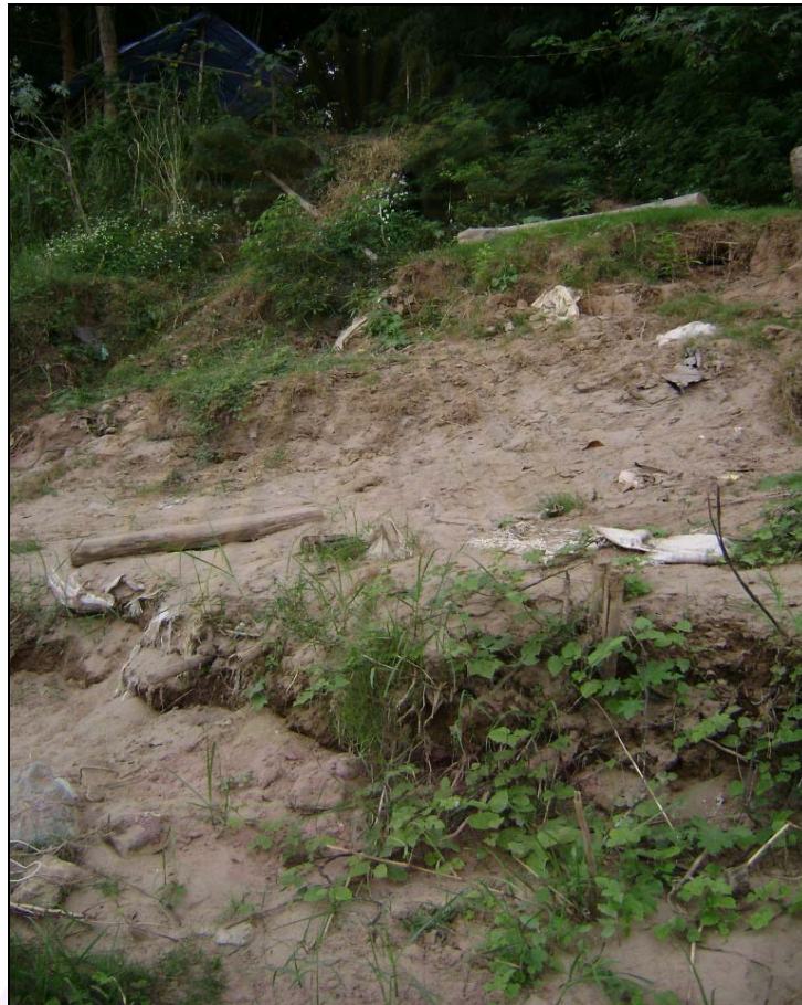
Figure 6: Soil erosion at Baan Pak Ing Tai
