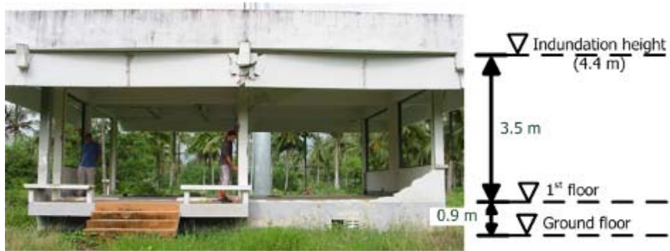
Figure 4-8. The former office of Thai Meteorological Department in Phang-Nga (Lukkunaprasit et al., 2010)
