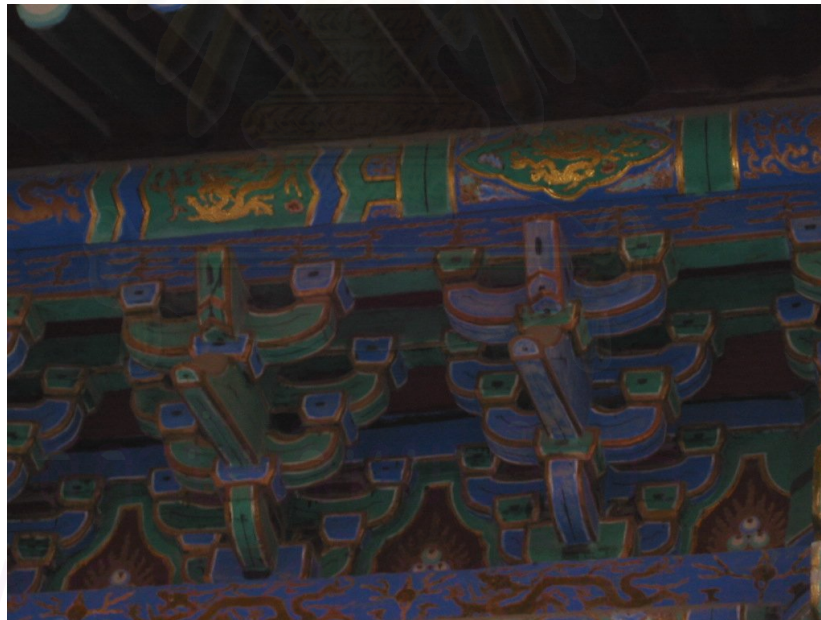
Pic. 19 b. The close-up view of the bracketing system in the east side of the three-tiered stage the Pleasant Sound Pavilion. Photo taken by Sasiporn Petcharapiruch on November 11, 2004.
