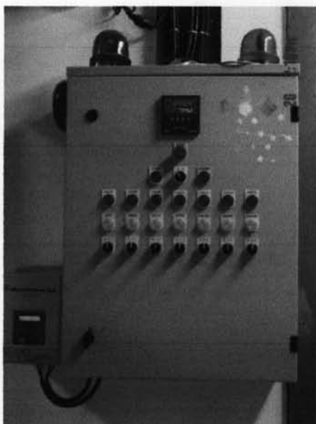
Figure 1: Furnace controlling system
