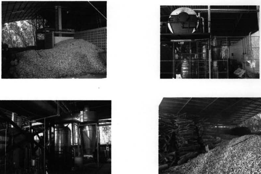
Figure 3.4: Furnace (fuel burner), boiler station unit, cyclone tank and fuels (firewood and corncobs)
