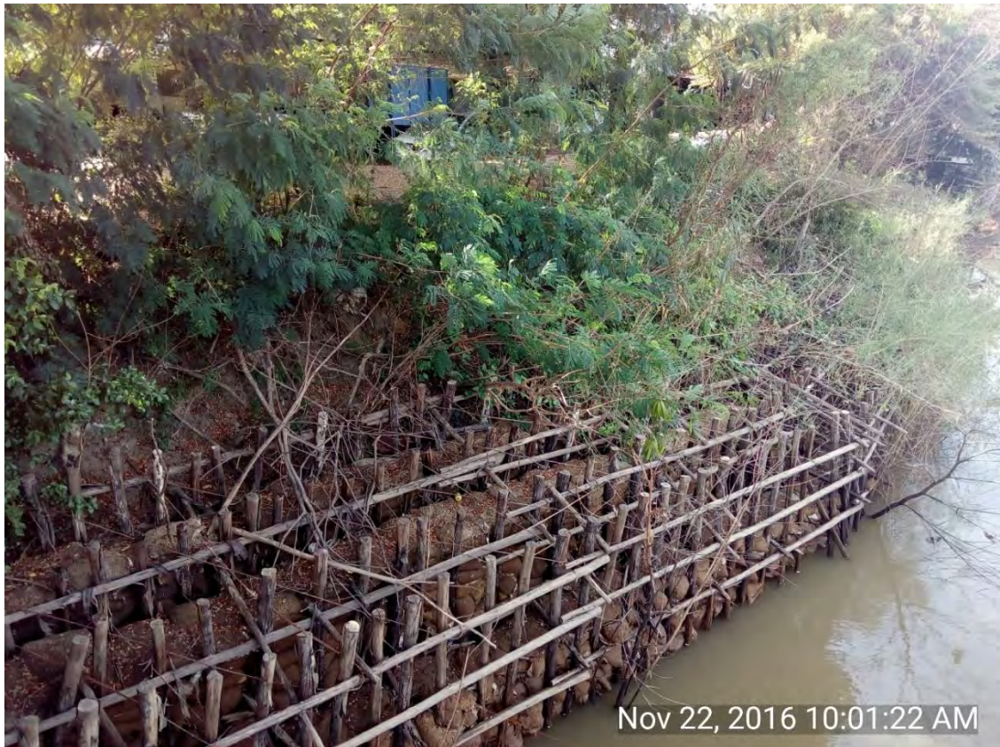
Figure 6. River bank failure protection alongside Bang Ban canal.
