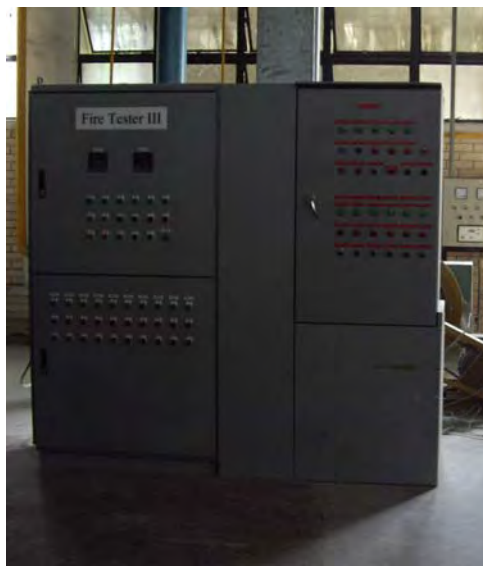
Figure 3.4 Controller of furnace
