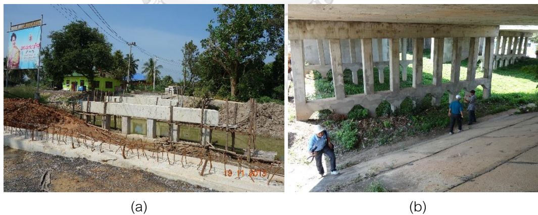
Figure 1.2 (a) Construction practices directly steel bar of columns to footings or cap beams (b) Bridge pier structure with a 10 meters span of the Department of rural roads (DRR), Thailand
