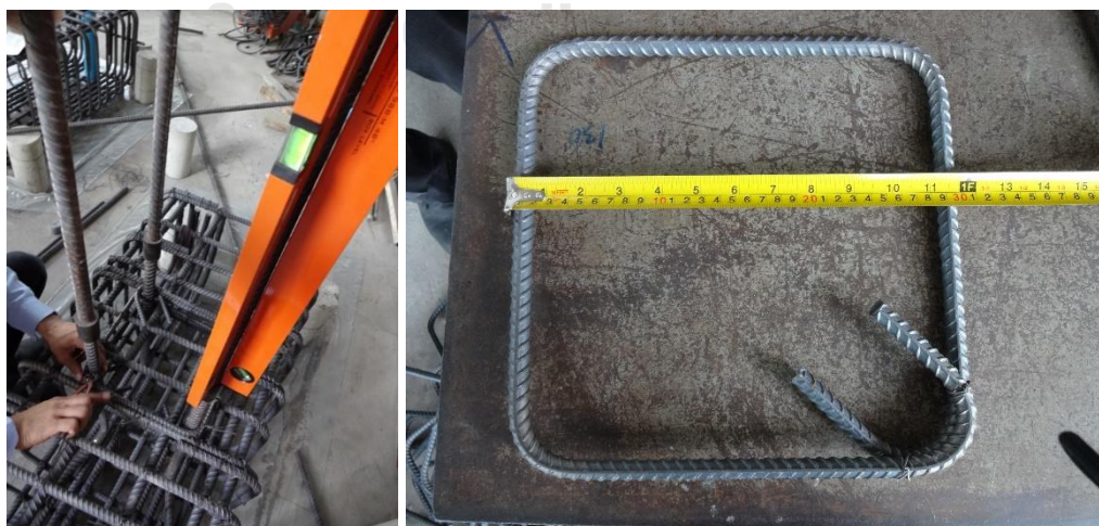
Figure 3.5 Tie hoops were placed orderly way along the column and vertical alignment was adjusted
