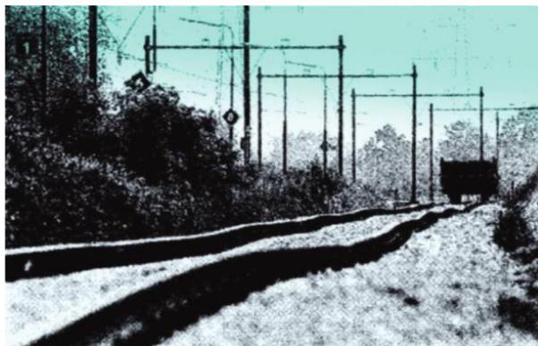
Figure 2.3 Differential settlement in rail track caused from the deformation of ballast (Indraratna et al., 2011).
