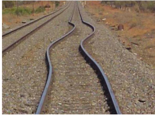
Figure 2.6 Track buckles because of lacking lateral confinement (Indraratna et al., 2011)
