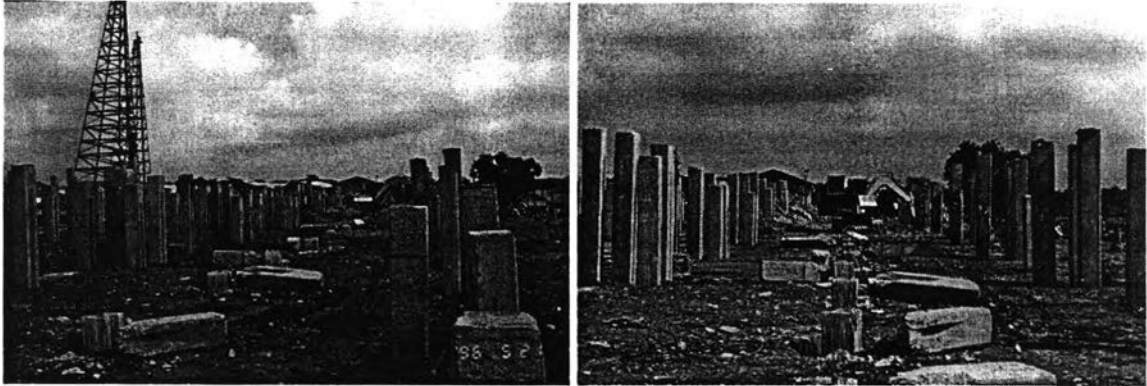
Figure 3.4: Driven piles obstruct operation of an excavator.
