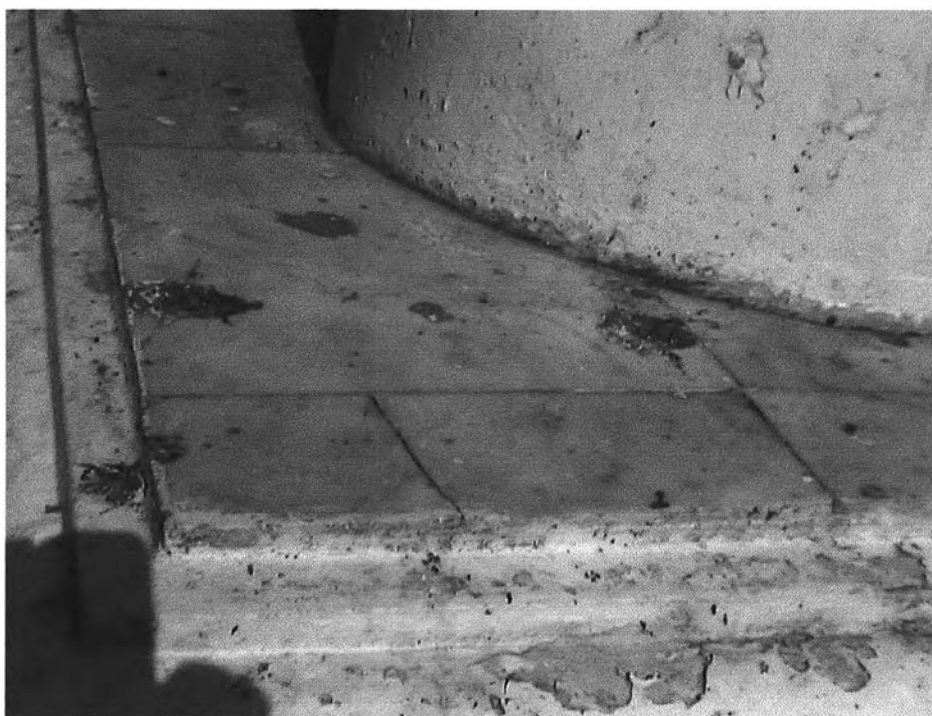
Figure 2 Pigeon droppings scattered on the side way around Wats.
