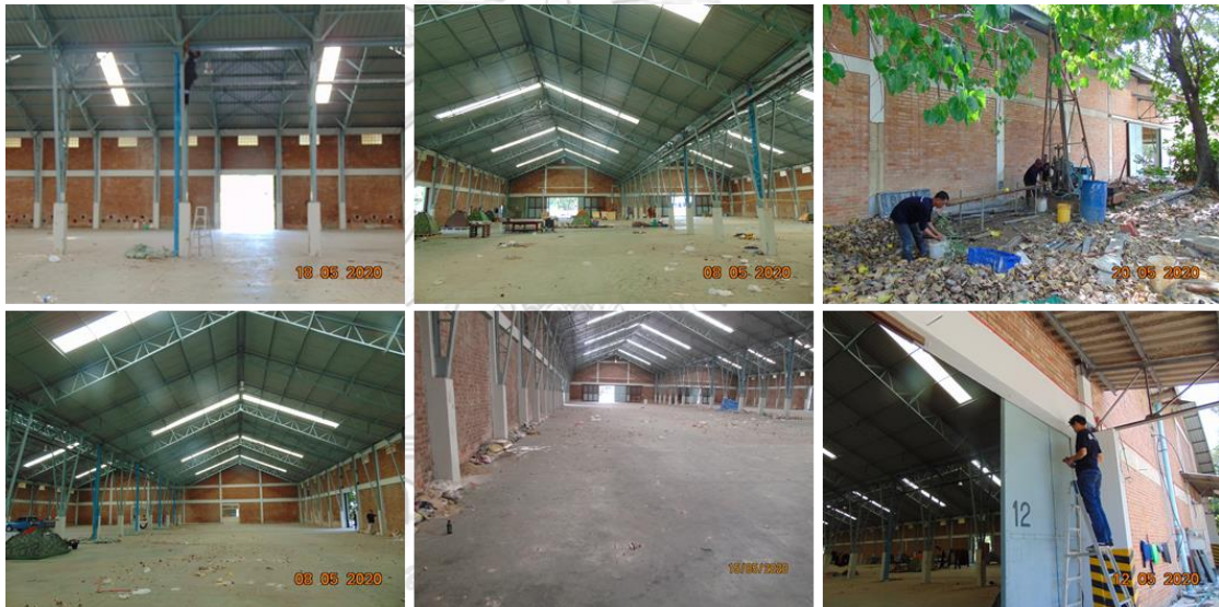
Figure 41. Overall realistic structure was inspected flaws in the research.
