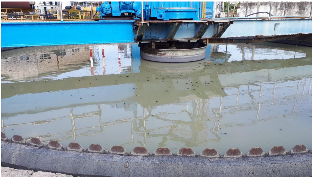
Figure E7 Sedimentation tank at WWTP B.
