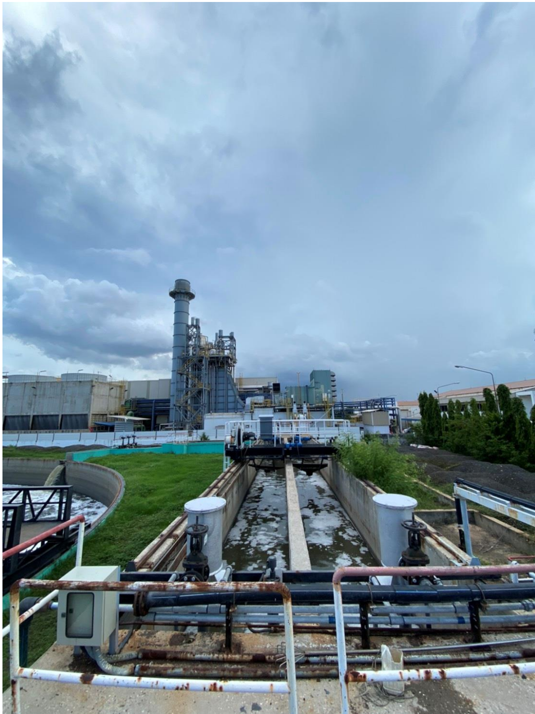
Figure E2 Grit chamber at WWTP A.
