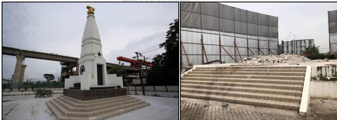
Photo 36. Pictures of the Constitutional Defense Monument in Laksi District, Bangkok Before and During the Demolition. Retrieved from (The Nation Thailand 2019).
