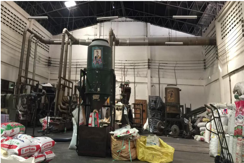
Fume extraction system of Plant B
