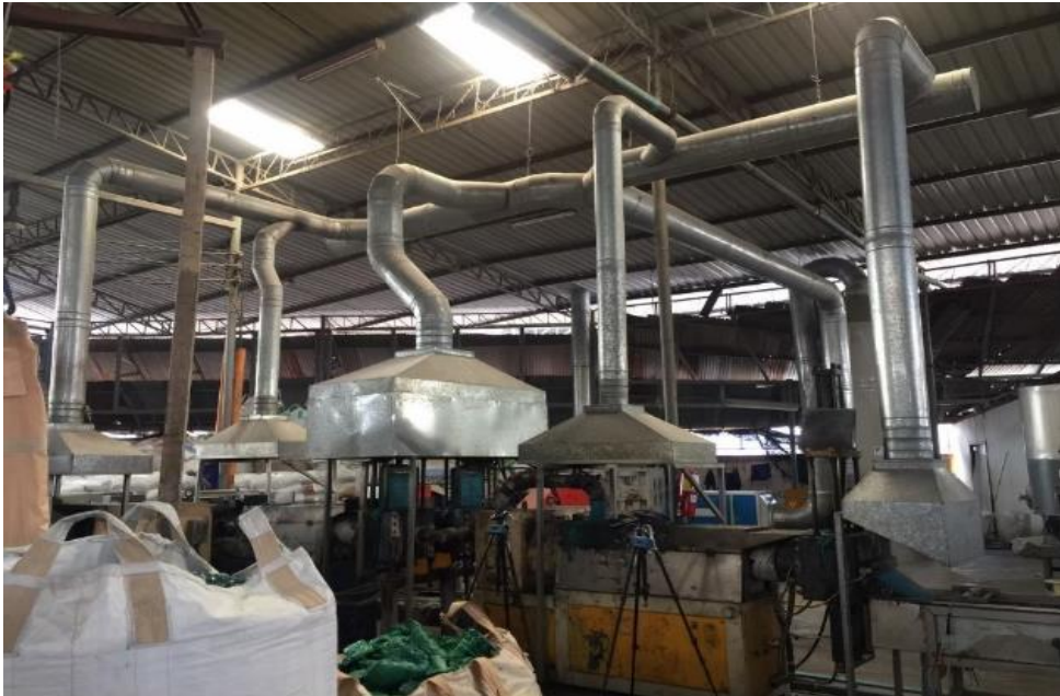
Fume extraction system of Plant A
