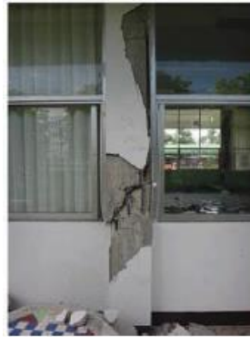
Figure 1.2 Shear failure on ground floor column Lukkunaprasit et al. (2015)
