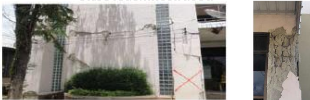
Figure 1.1 Soft first story with torsional irregularity and severe damage to the corner column Lukkunaprasit et al. (2015)
